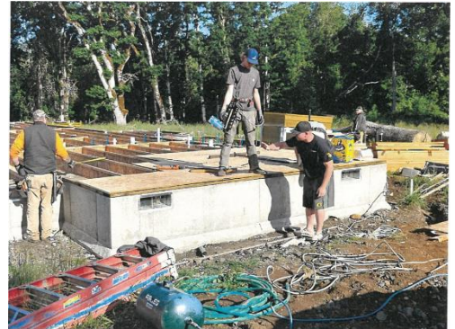
Boyd Rinck, owner of Coast Fork Construction giving some last minute instruction to his crew.
