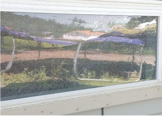
Recently shattered front window.
