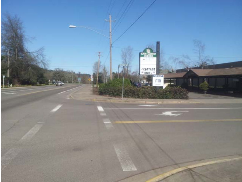
Fading Crosswalk Markings at Row River Road and Jim Wright Way
