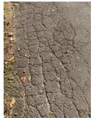
Poor Path Conditions
