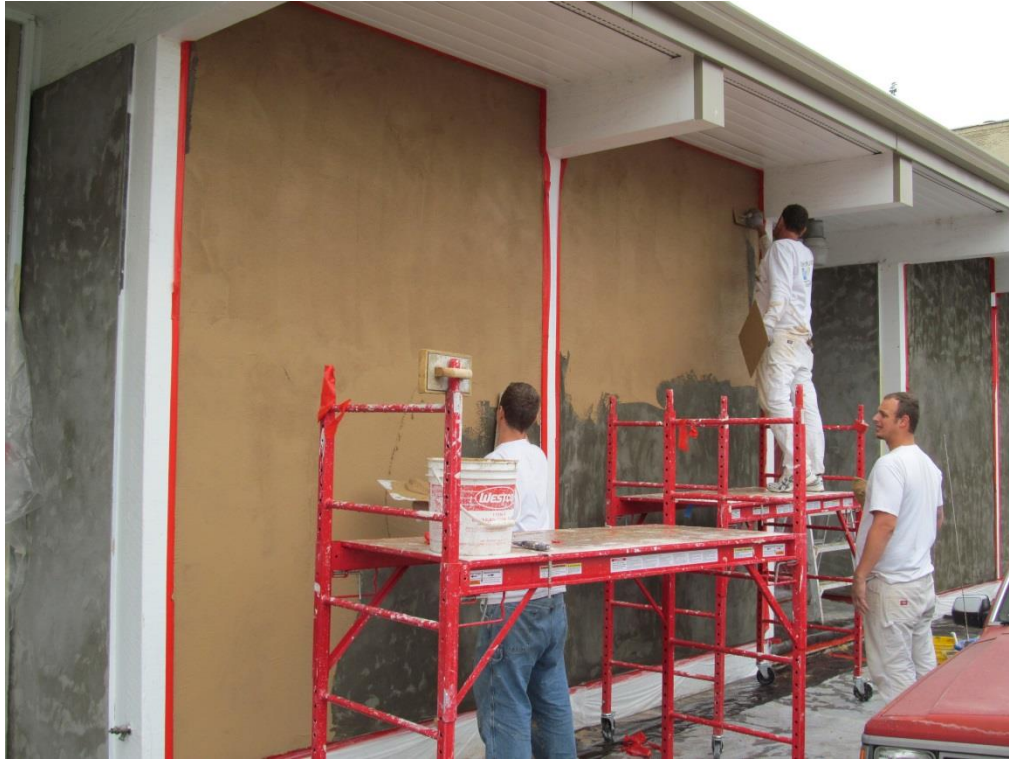
Ongoing restoration of 802 E. Main Street, funded through Historic Renovation Grant program, 2012.
