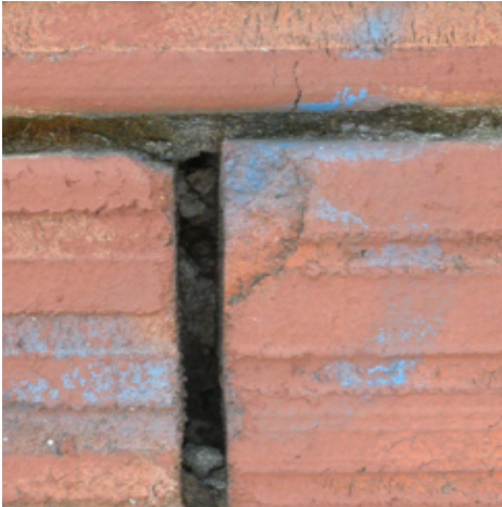
Figure 12. Open Joint with Deteriorated Mortar
