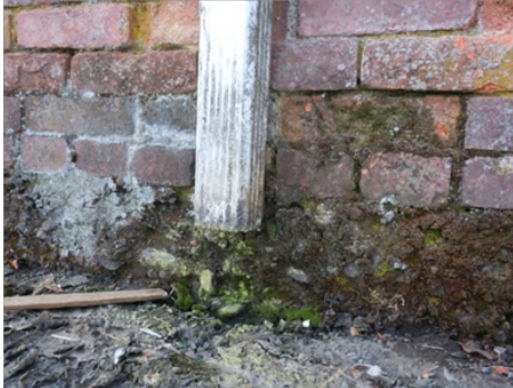
Fig. 19 Water is not being diverted away from the foundation of this building, causing rising damp
