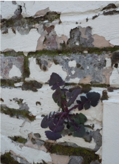
Fig. 21 Chipped paint is allowing water to enter into the joints of this brick wall
