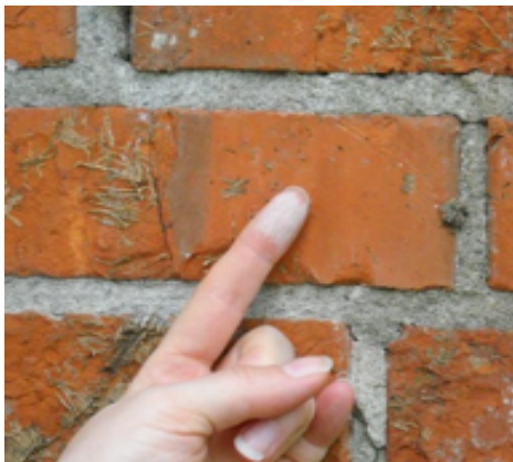
B) Chalky: significant lime present. This exterior chimney was built in 1928 in Eugene and likely uses a manufactured lime binder.
