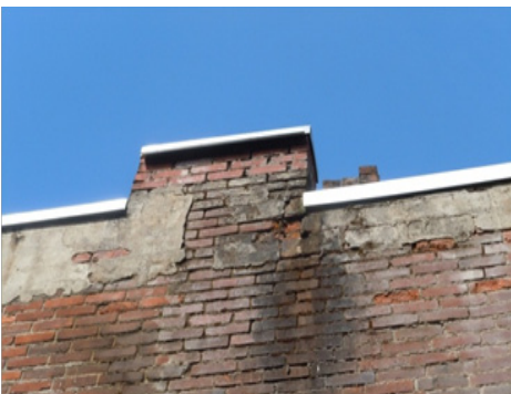
Fig. 18 Wall with flashing. Water being diverted away from parapet after years of damage from water infiltration.
