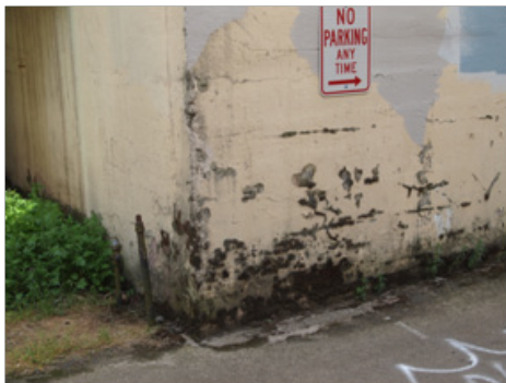
Discoloration/Stains: Improper Drainage
