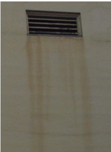
Discoloration from the Oxidation of Metal
