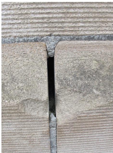
Figure 12: A compromised mortar joint has left the stone exposed to weather, resulting in spalling of the masonry.
