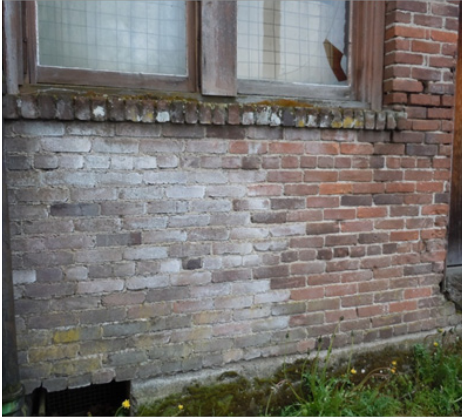
Fig. 22 Efflorescence on the surface of a brick wall
