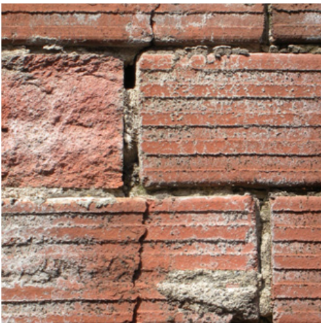
Figure 7. Cracked Terra Cotta.
