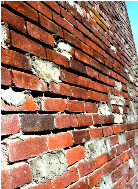
Fig. 30 Improperly replaced brick affects both the structural integrity and aesthetic qualities of an historic building
