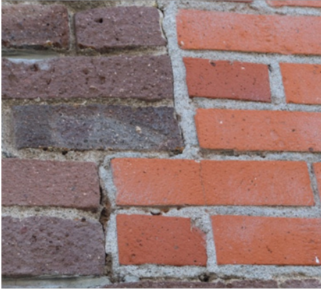
Fig. 24 Incompatible brick infill
