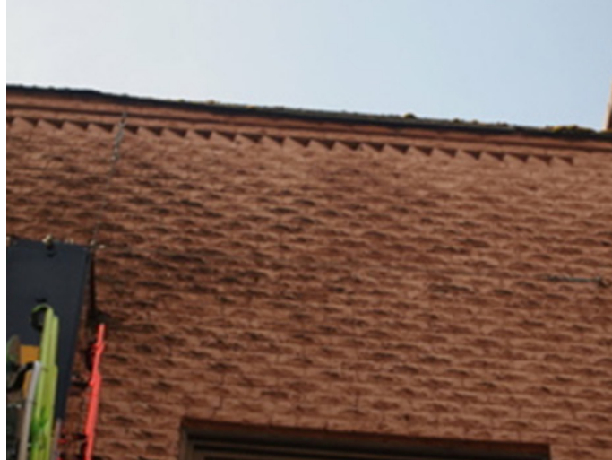
Figure 5: “Mousetoothing” near the top of the façade
