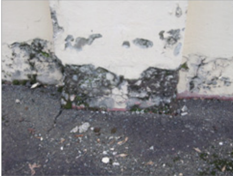
Coving: Repeated water Backsplash with resulting Spalling below
