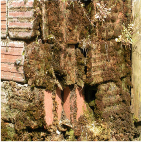
Figure 6. Severe Biological Growth and Deterioration of Terra Cotta.
