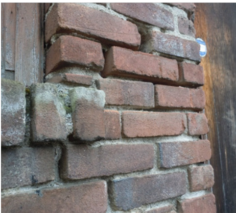
Fig. 27 Left untreated, the mortar gaps in this picture eventually cause structural damage to the building
