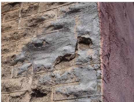
Figure 10: Inappropriate brick repair
