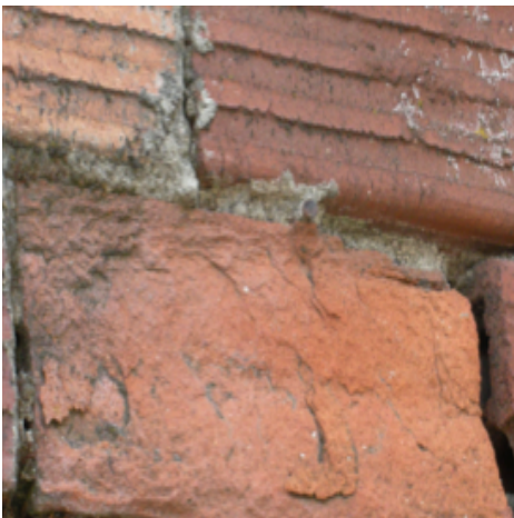
Figure 13. Spalling on Structural Terra Cotta
