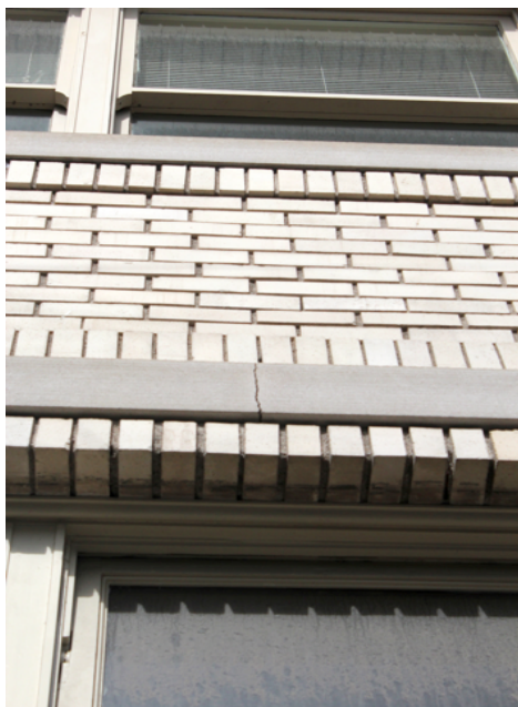
Figure 13: A vertically cracked lintel indicates horizontal settling of the building..
