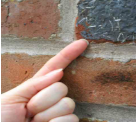
A) Clean: no lime. This exterior chimney was built in 1982 and uses a cement binder.
