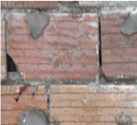
Figure 21. Improper Repair of Structural Terra Cotta
