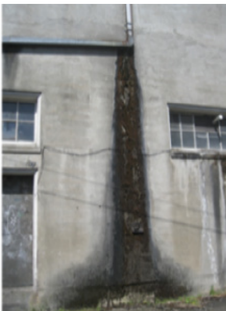
Plant Growth: Improper Drainage with Efflorescence on the right
