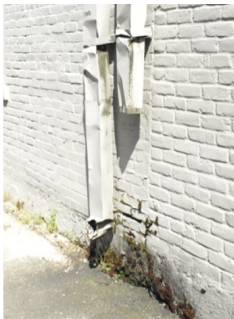
Water Drainage System
