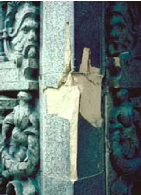
Figure 15. Material Spalling (Tiller 1979)
