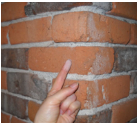
C) Very Chalky and Soft: natural lime. This interior chimney was built before 1900 near Cottage Grove. Its mortar easily crumbles to the touch.
