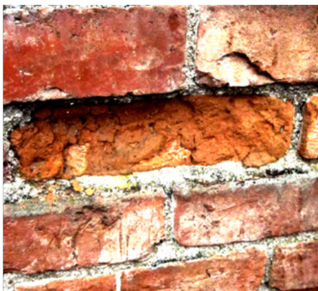
Fig. 29 Deteriorated historic brick unable to be reversed
