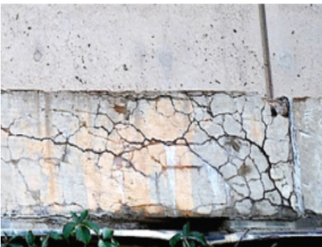
Possible Chemical Reaction Cracking, but laboratory tests are needed for verification
