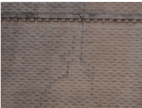
Figure 8: Step Cracking and other vertical cracks indicate horizontal movement
