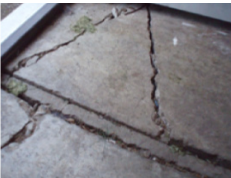
Cracking: Foundation Movement
