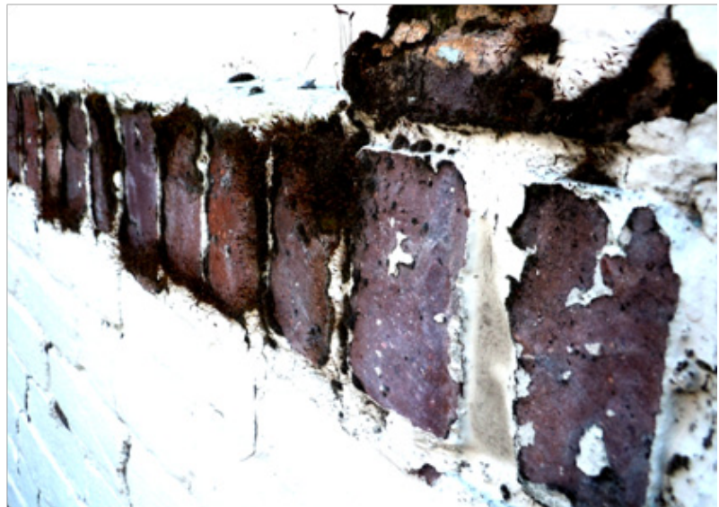
Fig. 11 Historic masonry painted with modern latex paint that will not stick due to water problems
