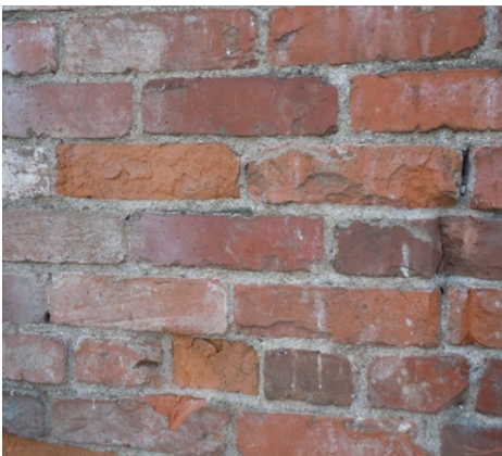
Fig. 23 Spalling and loss of mortar due to efflorescence
