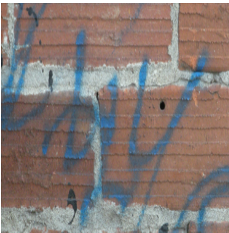
Figure 10. Graffiti on Terra Cotta Wall
