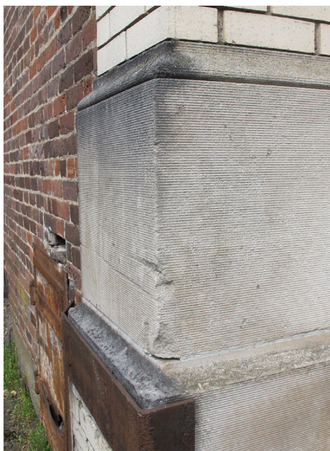
Figure 14: This stone plinth clearly shows soot accumulation as well as damage caused by passing vehicles.
