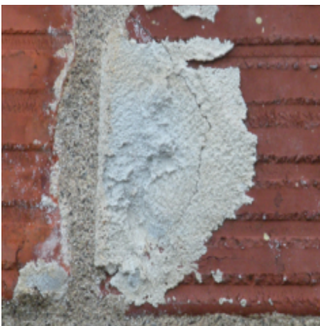
Figure 11. Improper terra cotta repair with incompatible material
