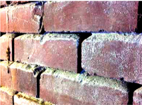
Fig. 28 Viable historic brick that needs repointing (www.indestructables.com)
