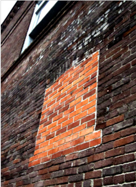
Fig. 12 Improper historic window infill
