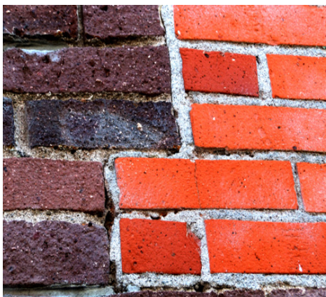
Fig. 9 Improper brick and mortar repair
