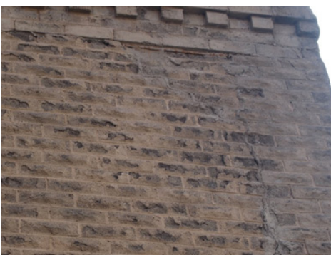
Figure 9: Spalling of rock-faced brick
