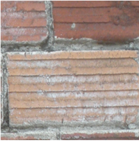
Figure 9. Efflorescence on Terra Cotta
