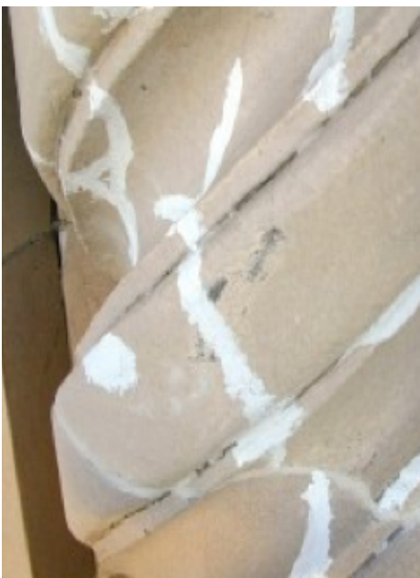
Figure 18. Cracked Terra Cotta Repair (www.preservationarts.net)
