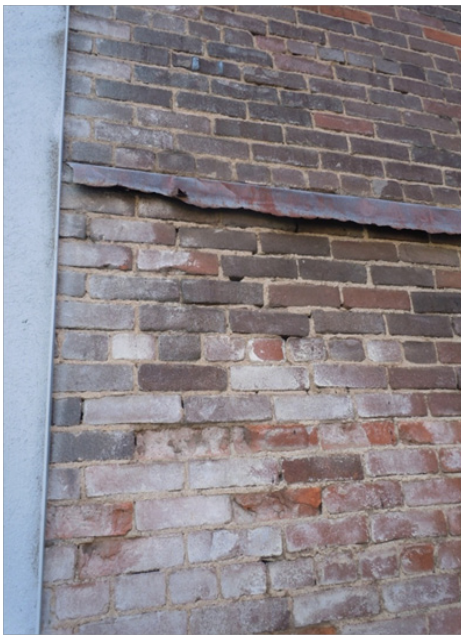
Fig. 20 Corroded metal imbedded in brick masonry
