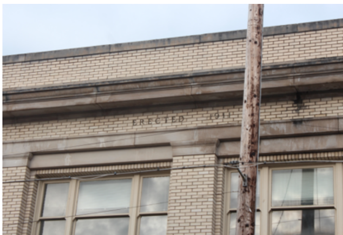
Figure 6: First National Bank Building – Close up of the cornice trim where it displays “Erected 1911”
