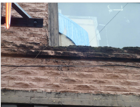
Figure 11: Biological growth can be seen on a large percentage of the front façade. A majority is underneath the windows indicating possible water drainage problems from the windowsills
