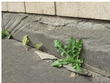
Figure 11: Coving from rainwater, resulting in delamination of the sandstone foundation. Plant growth also indicates moisture.
