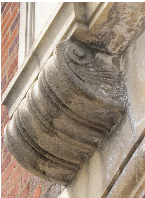
Figure 16: Efflorescence under the stone details of the door surround on the Volcanology building indicates moisture and salt movement through the materials.
