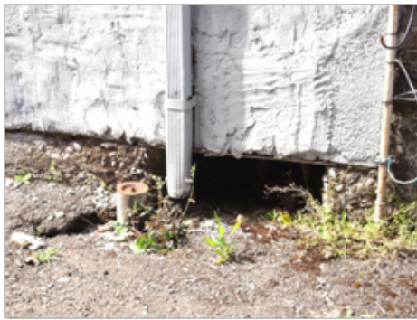
Cracking: Improper Drainage
