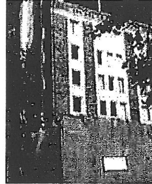
The lower floors of this historic brick and architectural terra-cotta building have been covered during chemical cleaning to protect pedestrians and vehicular traffic from potentially harmful overspray. Photo: NPS files.
