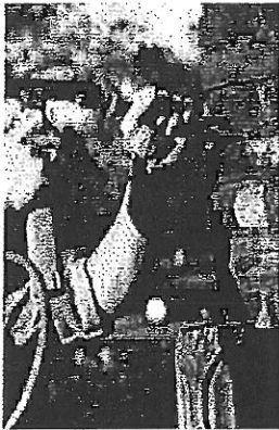
Here, a hammer and chisel are being correctly used to prepare a joint for repointing. Photo: John P. Spewilk.
