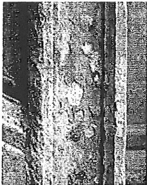
This clear coating has failed and is pulling off pieces of the stone as it peels. Photo: NPS files
