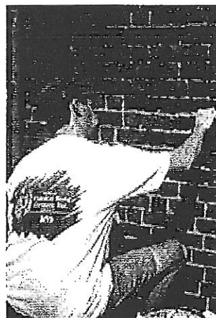
This early 19th century building is being repointed with lime mortar. Photo: Travis McDonald.
