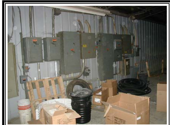
During the pilot test of its program, the Metropolitan St. Louis Sewer District concluded that this storage building was appropriate for wet flood proofing. The walls are metal and there is no insulation. The electrical service boxes would be moved above the flood protection elevation. The contents would be evacuated or moved to higher shelves when a flood warning is issued.
