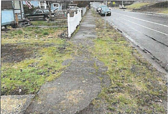
Figure 3-6. Example of Deteriorating Conditions on a Local Sidewalk
