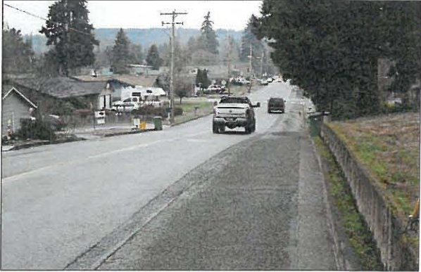
Figure 3-5. Sidewalk Gap on 6th Street
