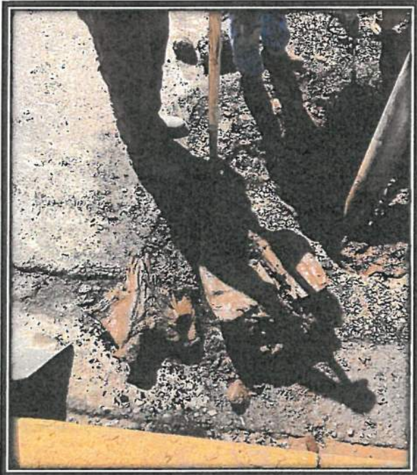
Sink hole on Gibbs caused by a rotten stump
