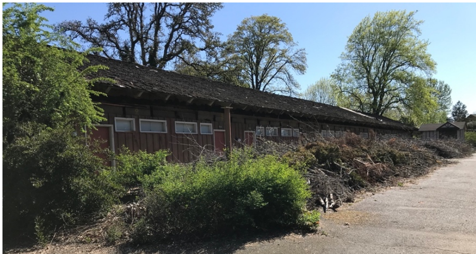
View of building in substandard condition when applicant purchased the site. The substandard buildings on proposed Lot 3 were demolished in 2022.
