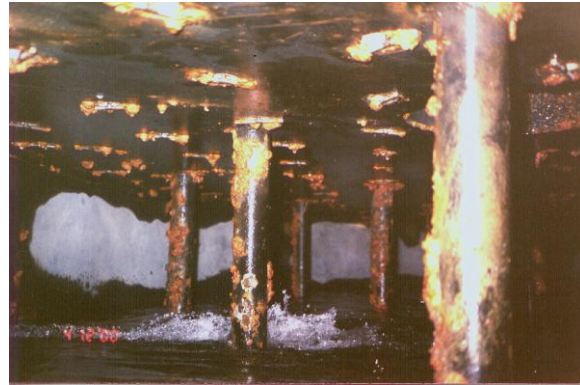
Space Below Filter Bottom
