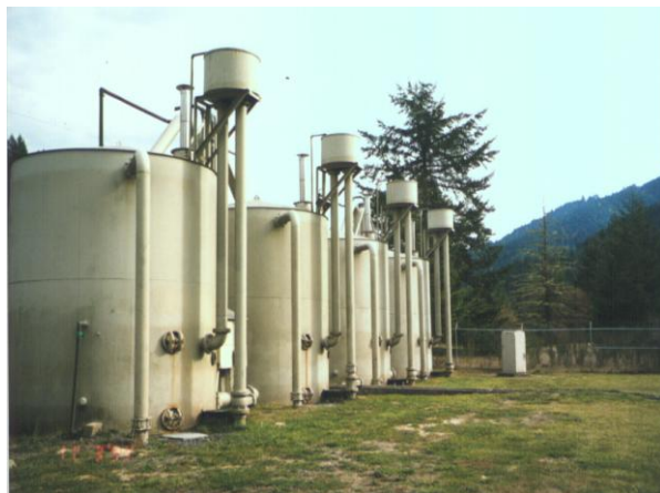
Filters at lower site
