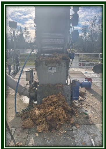
Sewer Treatment Plant plug from disinfesting wipes and rags
